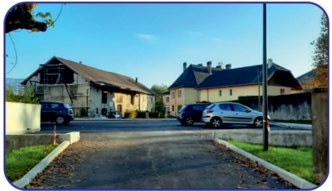
New outdoor car park built where the former vegetable garden was, opposite the entrance
